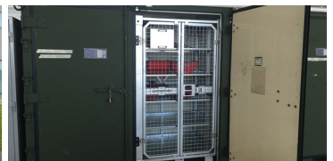
8145-01-512-1025 loaded in ISU90 with full access to gear
